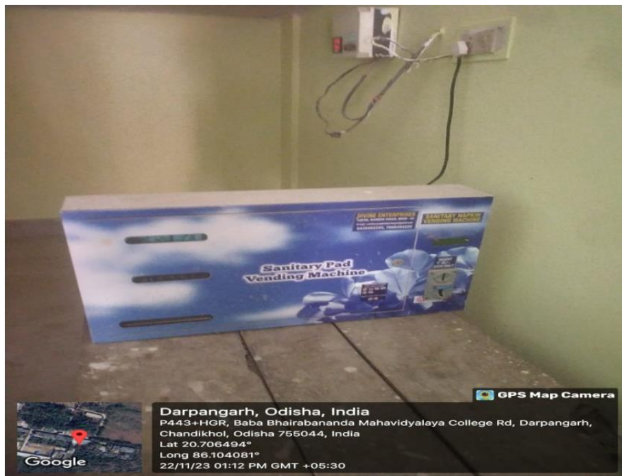
Figure-18: Installation of Sanitary Napkins Incinerator in Ladies Hostel
