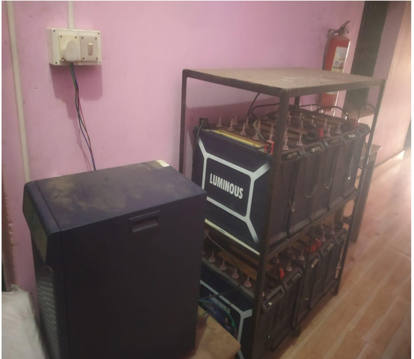
Use of Inverter in front of Principal Chamber
