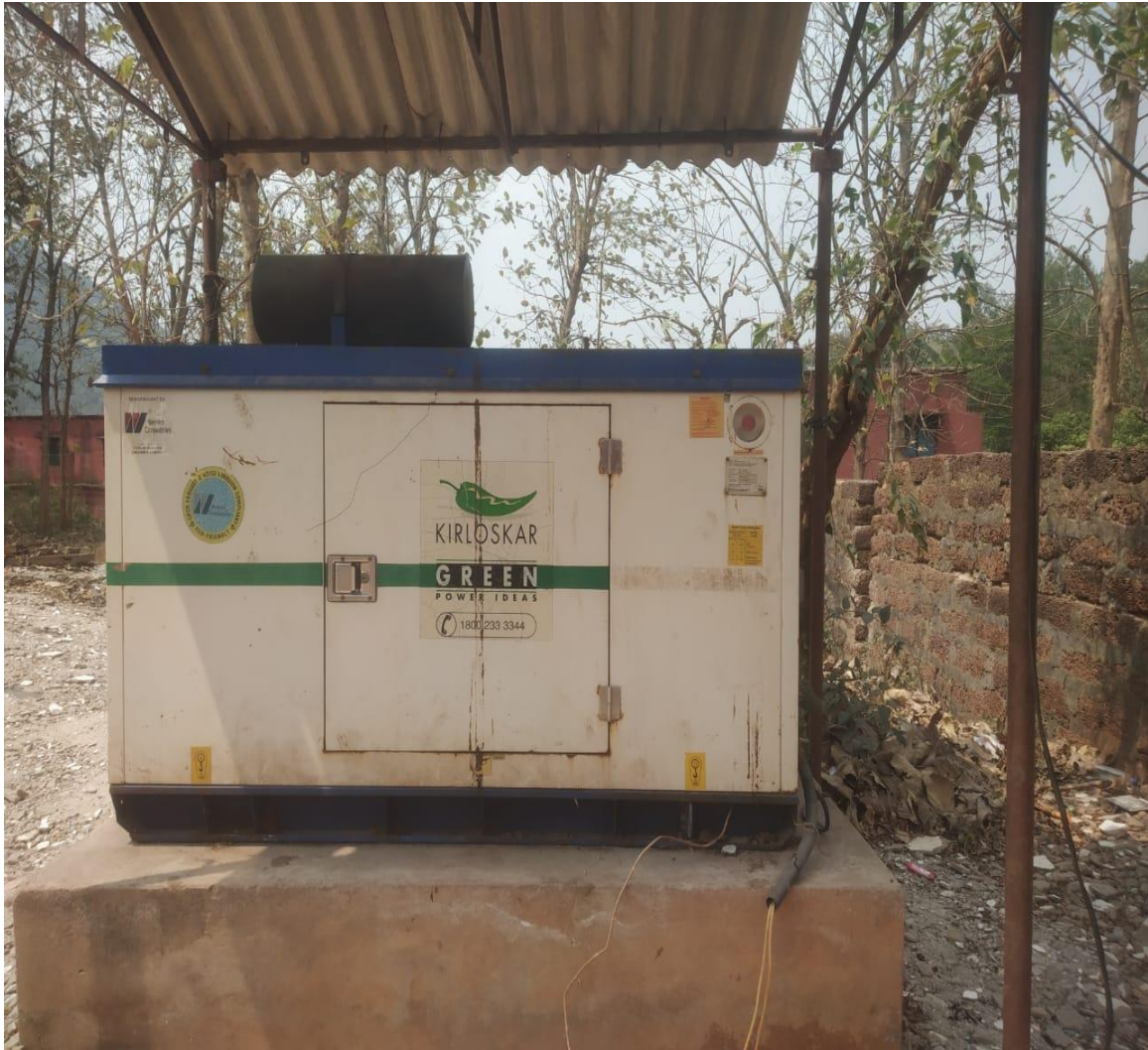
Diesel Generator at College Campus
